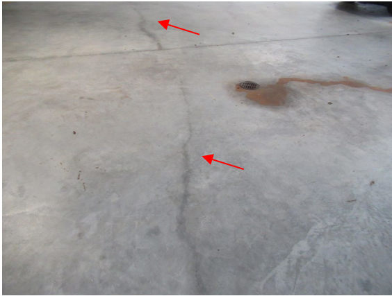
View of typical concrete topping shrinkage cracks.
