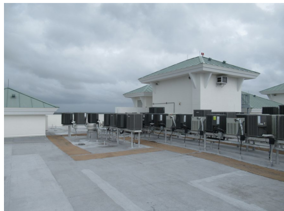
View of roof section and HVAC equipment.
