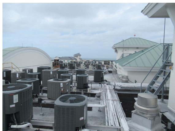
View of roof section and HVAC equipment.
