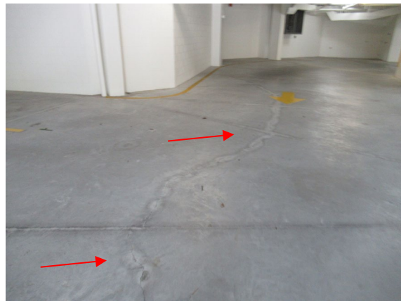
View of typical concrete topping shrinkage cracks.
