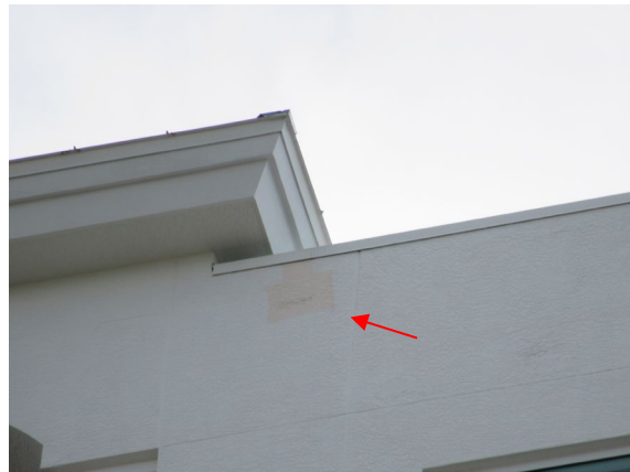
View of missed coating section on the western facade.
