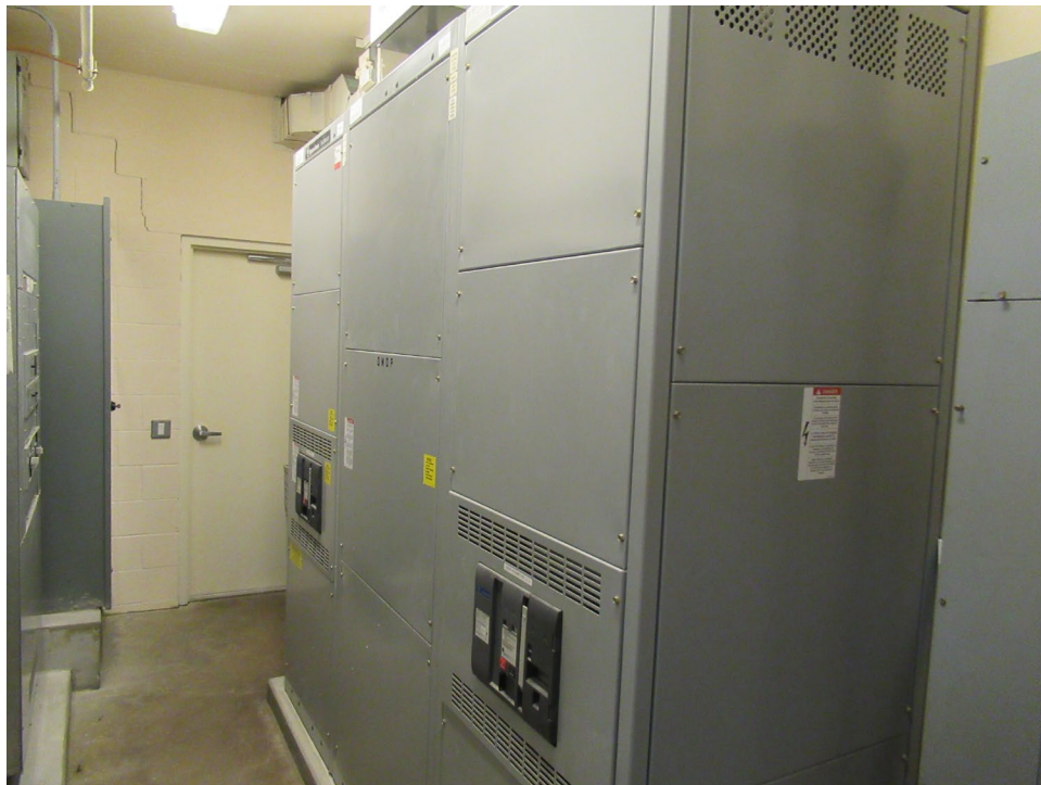
Photo 10 – View of electrical room equipment.
