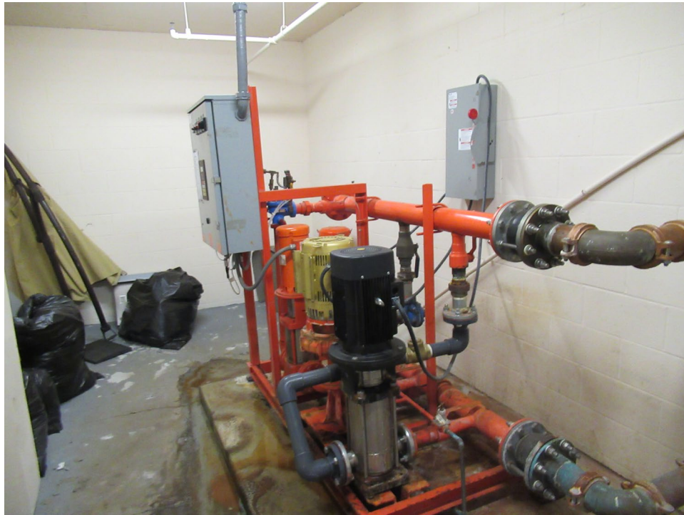
Photo 12 – View of fire pump.
