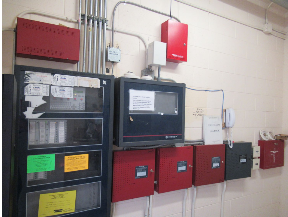
Photo 9 – Fire alarm control panel.
