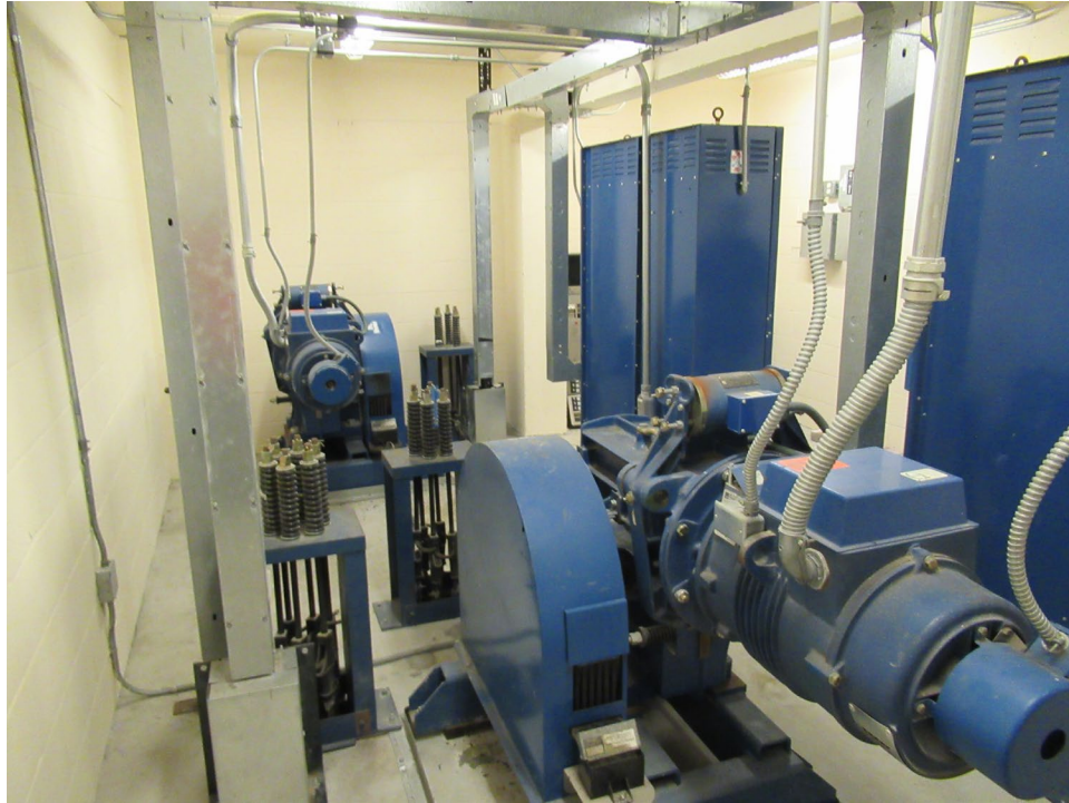
Photo 7 – View of elevator mechanical room.
