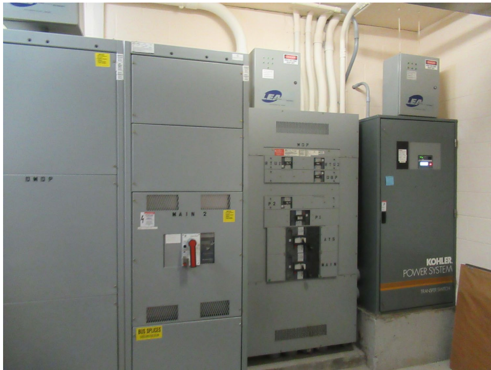
Photo 10 – View of electrical room equipment.
