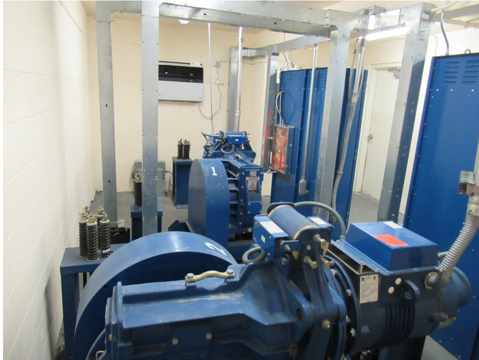
Photo 7 – View of elevator mechanical room.
