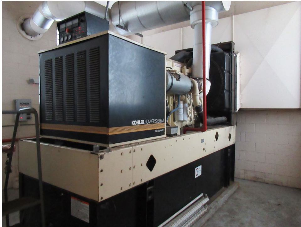
Photo 12 – View of electrical generator.
