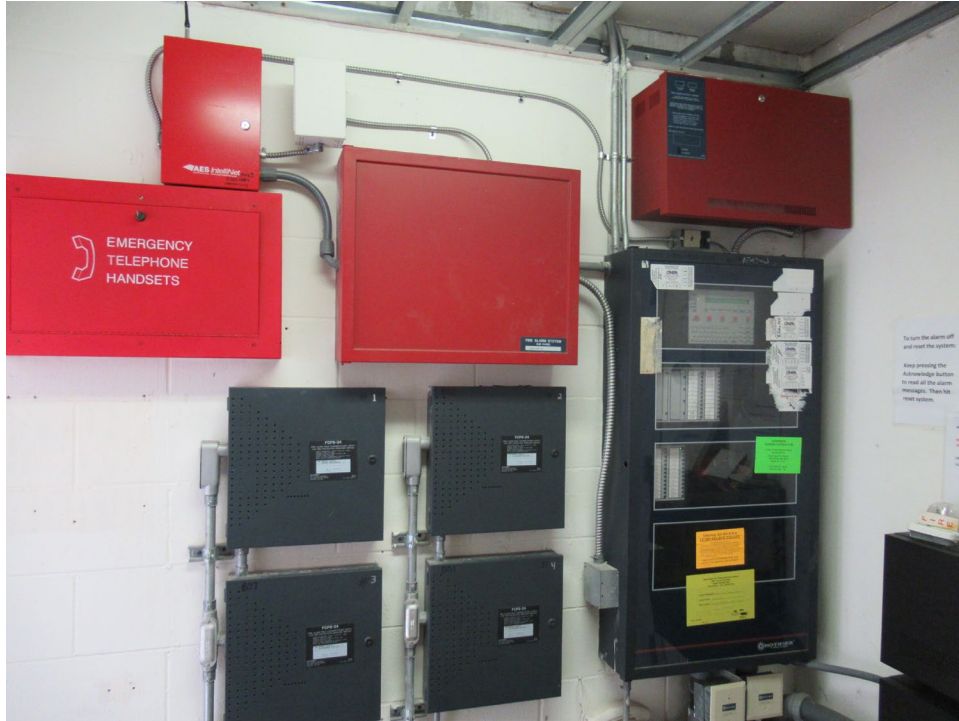
Photo 9 – Fire alarm control panel.
